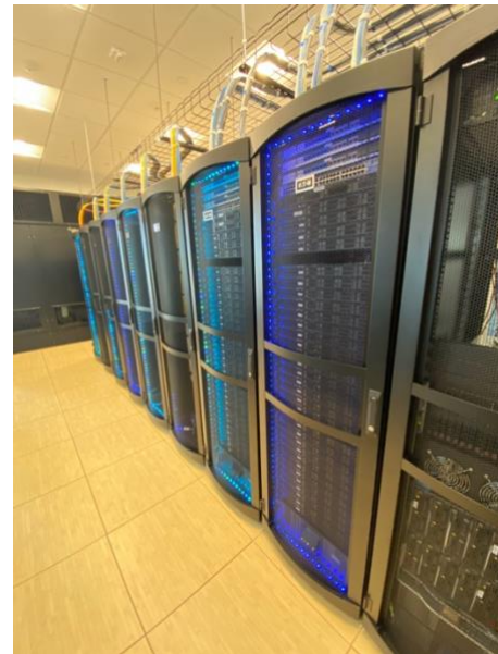
Figure 4 The front of the academic server room
