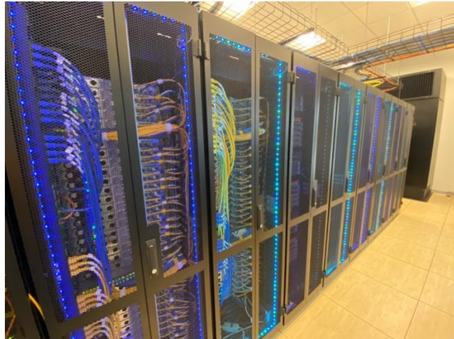
Figure 3 The rear facing academic server room
